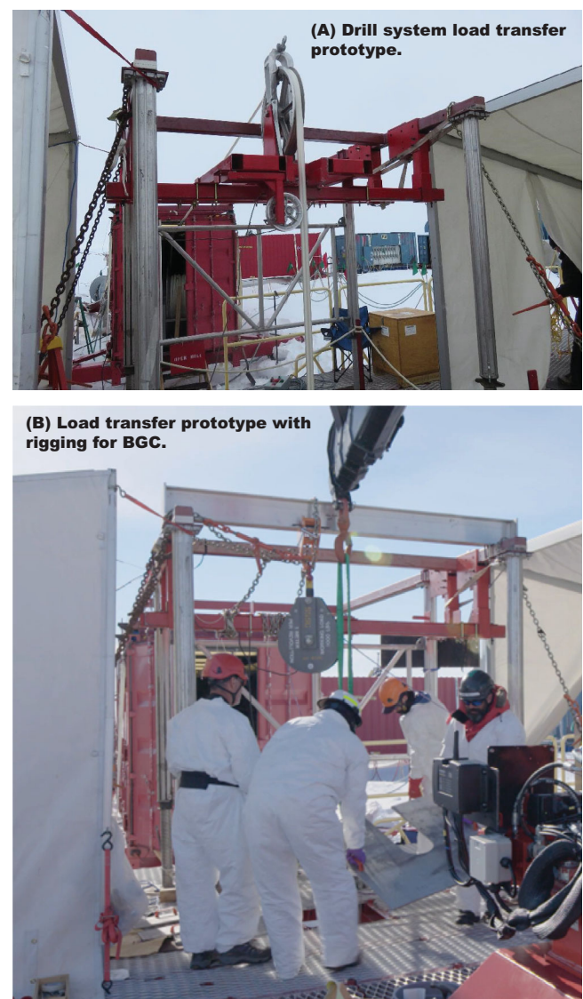
Fig. 5. Deck rigging for hot-water drilling and for scientific operations in the SLM borehole. (A) The prototype load transfer system was developed by the University of Nebraska hot water drill team to reduce transfer time between hot-water drilling and science operations. The system allowed the drilling mechanism to remain in place during science operations for ease of reaming (adding energy to the borehole to slow freeze-back). All scientific equipment was deployed and retrieved from this rigging using a custom-built winch and metering block assembly (the smaller sheave oriented perpendicular to the large upper one deploying hot water drilling hose in (A) ), except the autonomous vehicle and the BGC. (B) For the heavier weight of the BGC, an aluminum I-beam (top) was added to the load transfer main frame. The sheave was mounted on this I-beam with a beam clamp and positioned over the center of the borehole with tension (when the sheave is at approximately 45° angle). In the photo, the BGC is at the surface of the borehole and the crane is positioned overhead for load transfer after temporarily supporting the corer on the bracket being employed by the two people in the foreground.
